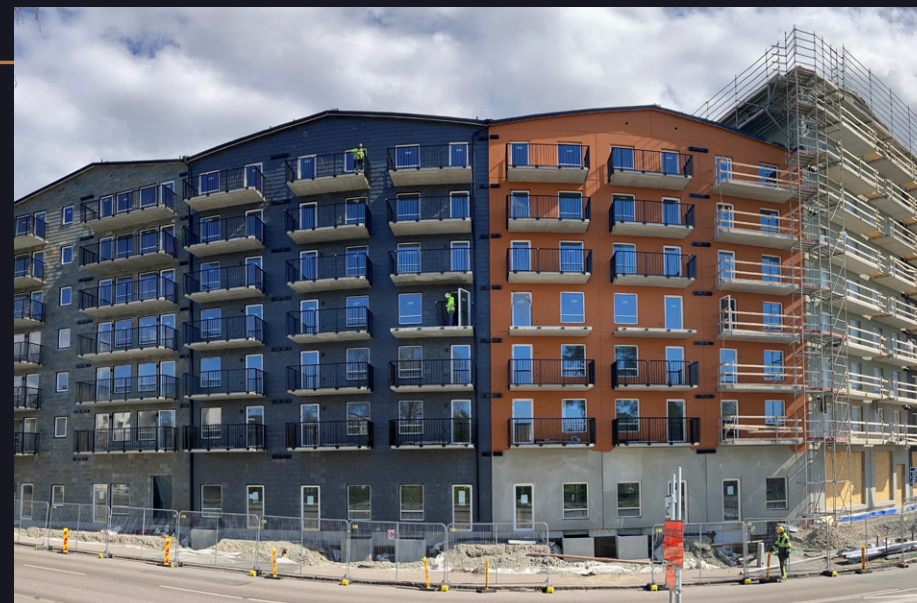
Our construction of 103 Lateral Low-Rise apartments on Smörslottsgatan in Gothenburg is starting to take shape. Tenants are scheduled to move in during December 2021.
